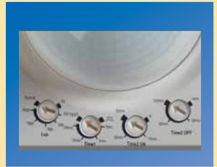
Simple lux value and time setting with protective cover against unauthorised adjustment. HVAC channel switches on presence dependent basis with on/off switch delay, producing particularly efficient operation.
